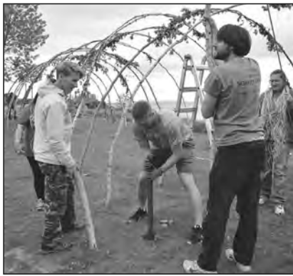
Thomas Walser, centre, works on the hole in which a sapling will be secured to become part of the teaching lodge structure at Marina Park while, from left, Laura Ojala, Dave Nagy, Dave Bates and Patti Whitcowl look on.
